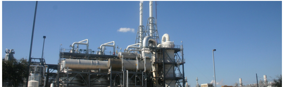
Waste incinerators and coal fired power plants rely on DioxSorb® powdered activated carbons for achieving their emission control goals.
